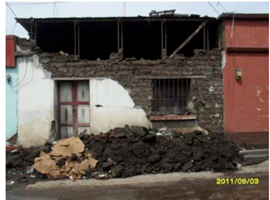
House of adobe mud and Straw destroyed by the earthquakes and daily tremors in Santa Rosa. Photo/Ana Paxtor con Cedepca
